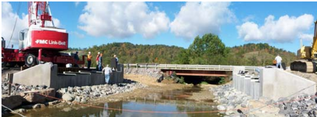
Abutment 1 (left) used SCC for its three caissons, while Abutment 2 (right) used a traditional caisson mix.
