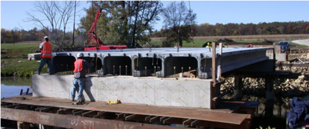
Ultra-high performance concrete was used in beams of the Jakway Park Bridge.
