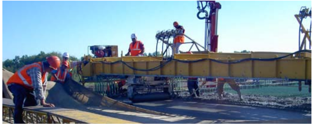
Wet burlap is placed within 10 minutes of strike-off for LC-HPC bridge decks.
