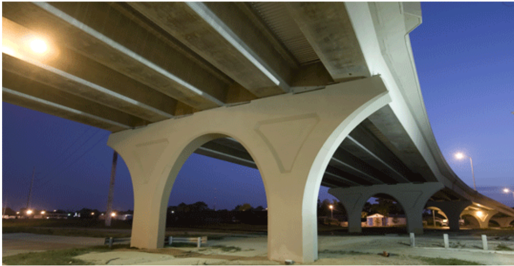
High strength concrete was used in the U-beams of the North Boulevard Bridge.
