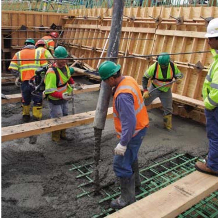
Casting the bottom flange of the cast-in-place superstructure. Photo: Tim Davis, FIGG
