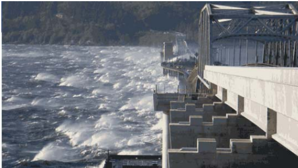
High performance concrete was specified to resist the harsh salt environment of the Hood Canal.
