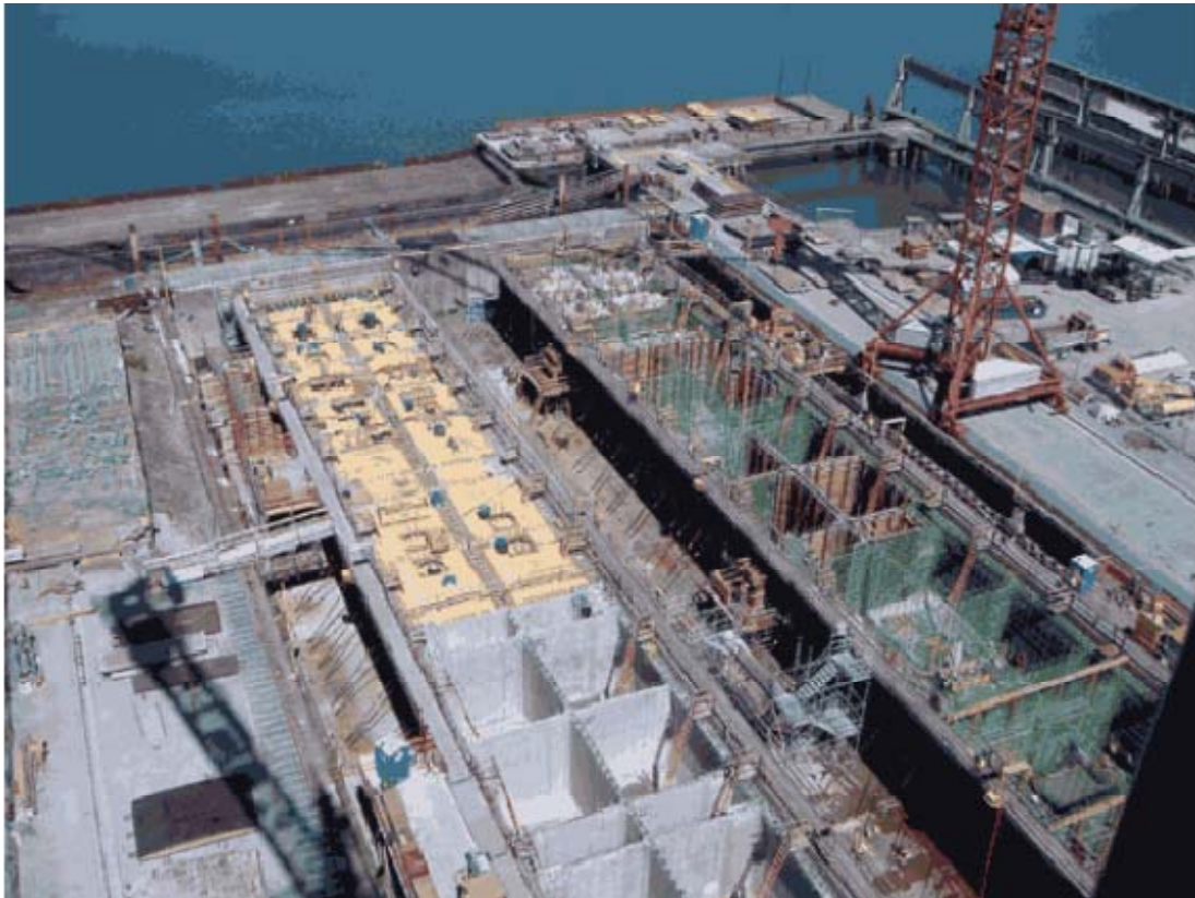
High performance concrete with a flow of 23 in. (585 mm) and a compressive strength of 11,000 psi (76 MPa) was used to cast the pontoon walls.
